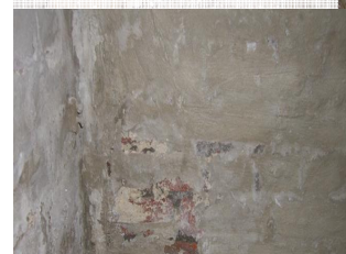
Area of failed tanking
