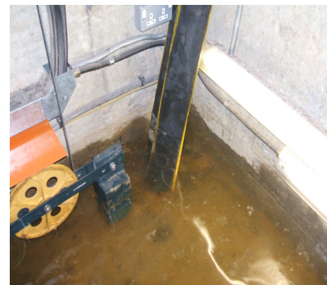
Standing water in a lift pit
