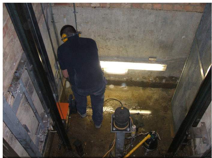
Standing water in a lift pit
