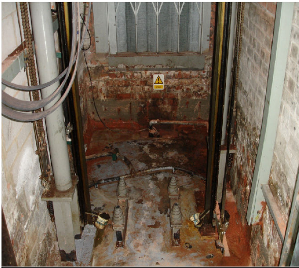
A lift pit showing signs of water ingress
