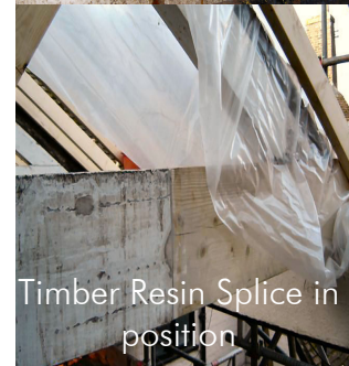
Original damage to trusses
