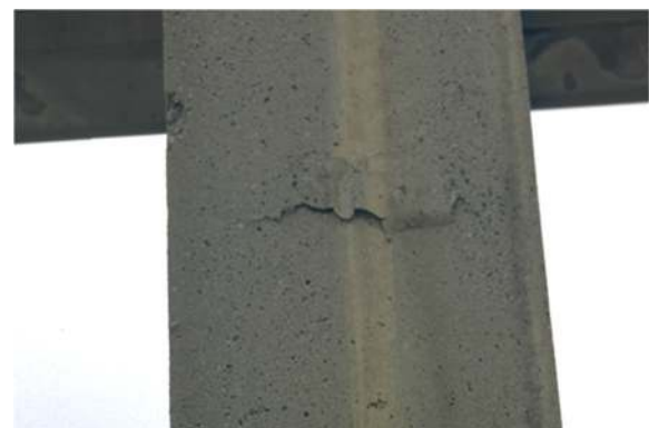
Reinforcement corrosion due to loss of pH-value of the concrete
