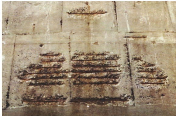
Corrosion through insufficient concrete
