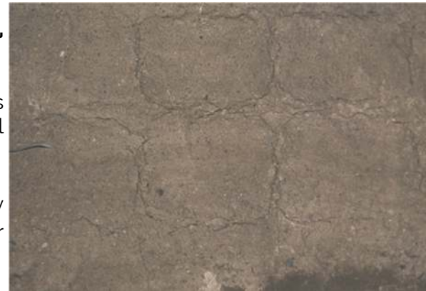
Cracking caused by sulphate attack
