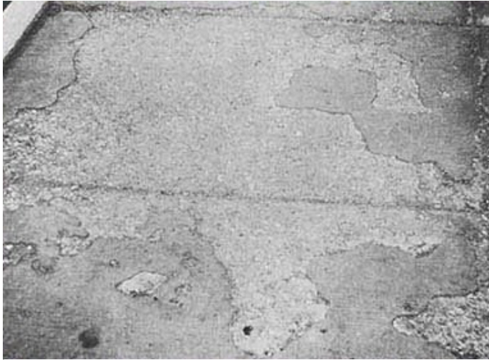
Damage caused by Freeze & Thaw
